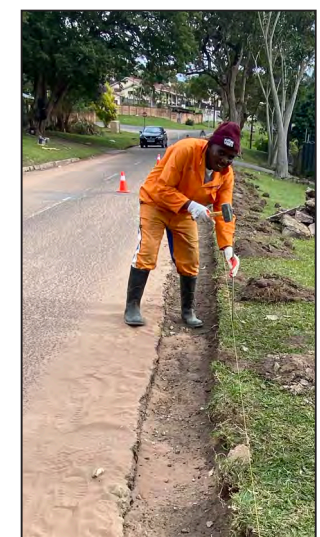
Teams from the City are hard at work in Ward 18 to install kerbs on Nelson Road, Finingham Ridge in Pinetown. Picture: MLUNGISI DLAMINI
