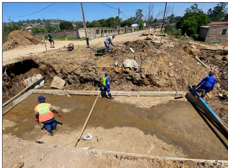
Repairs to Gogovuma Road in the uMzinyathi area in Ward 108 will ensure the smooth flow of traffic in the area. Picture: MLUNGISI DLAMINI
