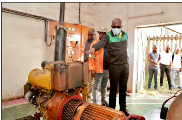
To ensure that all Durban beaches are operational ahead of the festive season, eThekweni Mayor Councillor Mxolisi Kaunda and Deputy Chairperson of the Human Settlements and Infrastructure Committee Councillor Bheki Mngwengwe conducted an oversight visit to Warner Beach and the Kingsway pumpstations. Picture: PUMLA KHWELA
